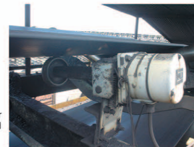
Conveyor Starting Indicator for indicating conveyor started
