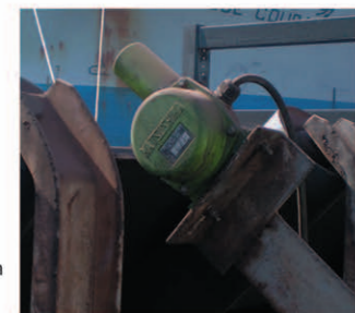
Speed Relay for conveyor slip detection
