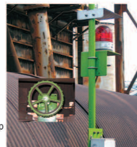
Pull Cord Switch for emergency conveyor stop
